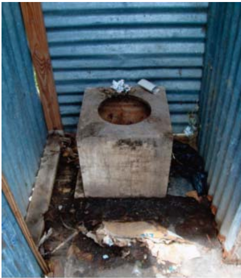
View down inside toilet seat.
