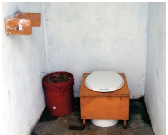
Figure 3: Toilet contents are covered inside the receptacle with sawdust and/or bagasse. The 20-liter receptacle simply lifts out when full.
